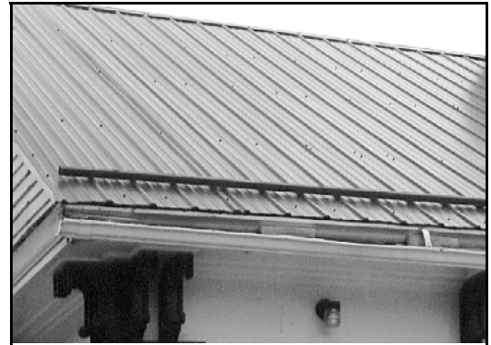
Commercial buildings with metal-clad roofs should have snow guards, brakes or other devices to prevent snow and ice shedding onto public ways.
