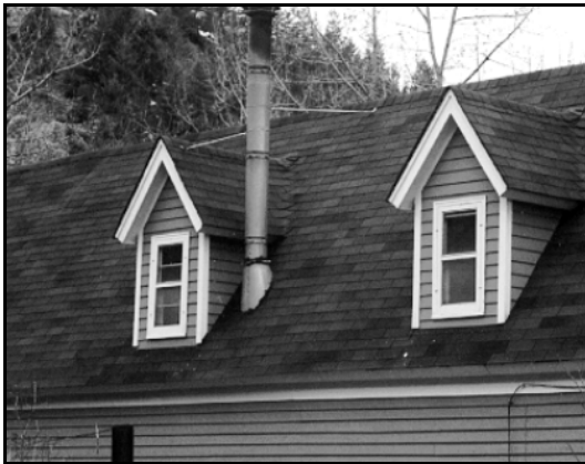
A new dormer should be lower than the primary ridge line and set in from the eave.
