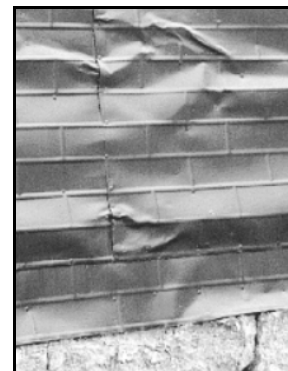
The historic stamped tin on the Georgetown Energy Museum is an architectural metal worthy of preservation.
