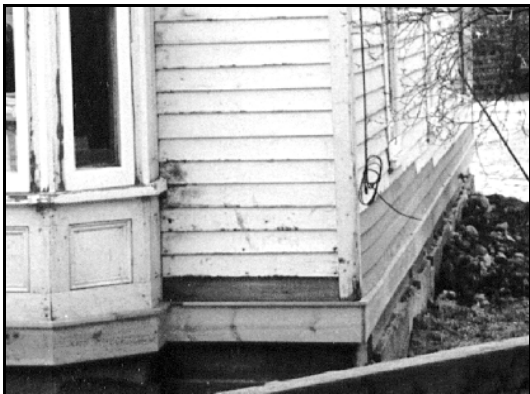
Repair wood features by patching or piecing-in new wood elements that match the original.
