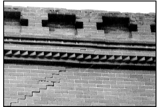
Preserve masonry features that define the overall historic character of the building,
