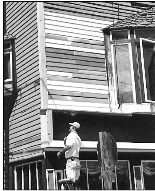
Materials should be applied in a manner similar to that used historically.
