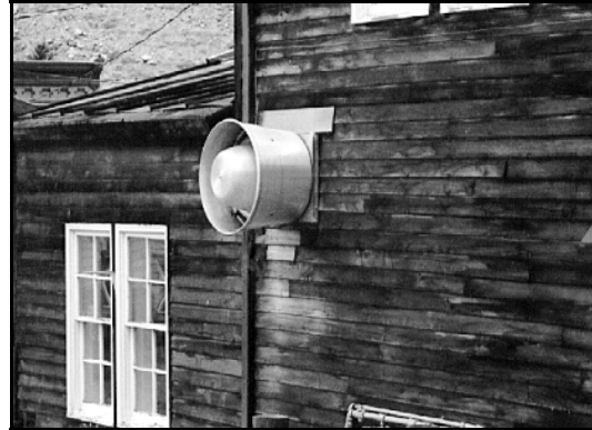
This exhaust fan is not integrated with the building and is inappropriate.
